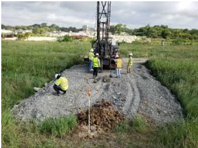
Photo #9 View of drill rig set up at boring location MM-3b with the methane monitoring point installed at location MM-3 in foreground. Note that MM-3b is being drilled through the soil access ramp (gray clay and shale) constructed for site access for this project.
