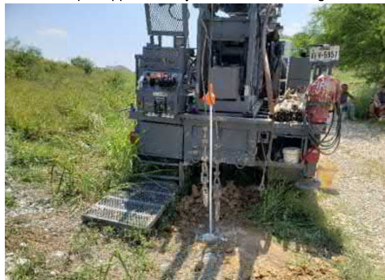
Photo #12 View of methane monitoring point installed at soil borings MM-4.
