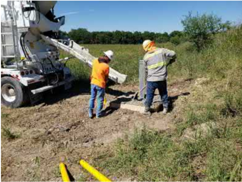
Photo #17 View of technicians installing protective boxes and concrete pads at methane monitoring point MM-2.
