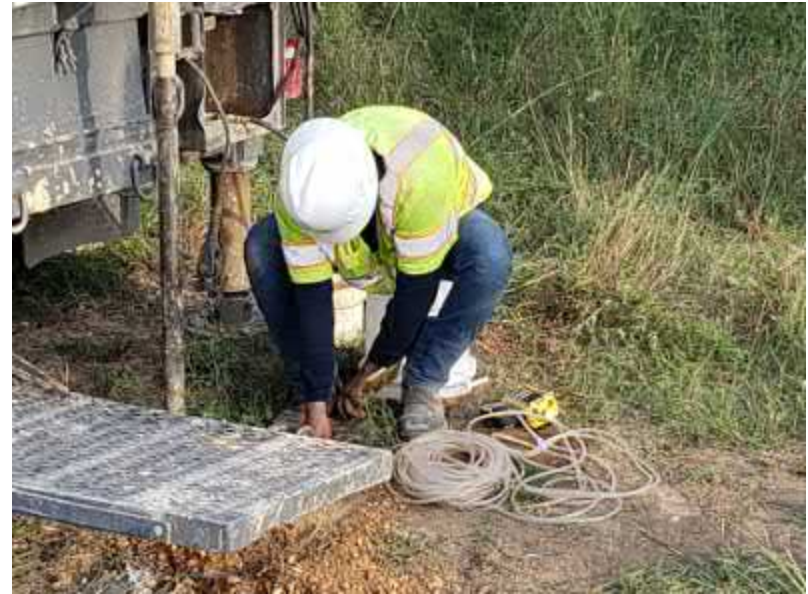
Photo #14 View of technician taking down-hole methane gas readings in soil boring MM-5.
