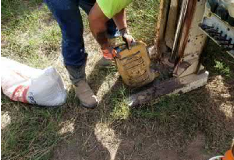
Photo #21 View of technician backfilling soil boring B-8 after drilling activities were completed.
