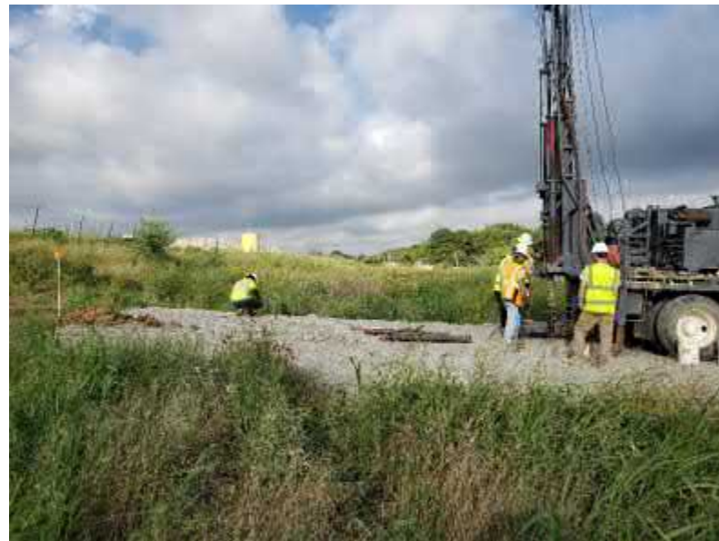
Photo #10 Another view of drill rig set up at boring location MM-3b with the methane monitoring point installed at location MM-3 is visible in the left-side of the photograph. Gray soil access ramp is approximately 3 feet thick under rig.
