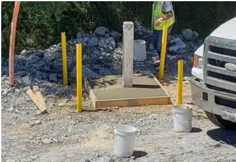
Photo #27 Typical view of completed methane monitoring point and well pad installation. Installation of protective bollards (yellow poles) was completed the following day.
