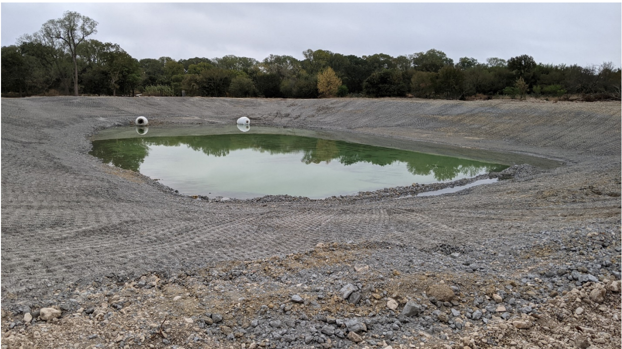
PHOTO 14 VIEW OF A MAN-MADE, RETENTION POND (WB005). WB005 WAS IDENTIFIED AS A MAN-MADE RETENTION POND EXCAVATED IN UPLANDS AND IS NOT LIKELY TO BE CONSIDERED A POTENTIALLY JURISDICTIONAL WOTUS. PHOTOGRAPH IS FACING NORTHEAST.
